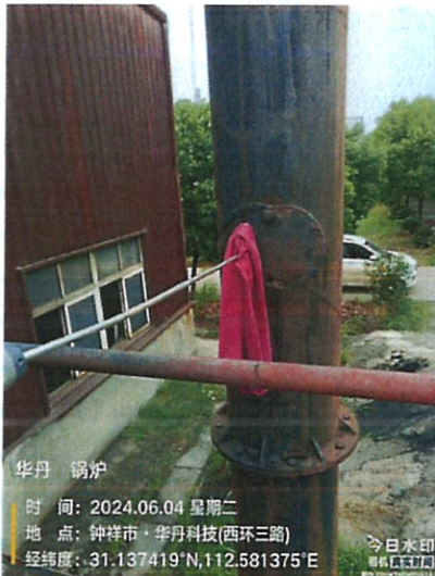
◎1 DW001 锅炉废气排气筒
